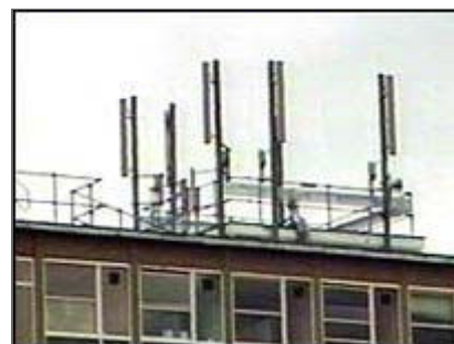
Typical roof mounted stub masts
